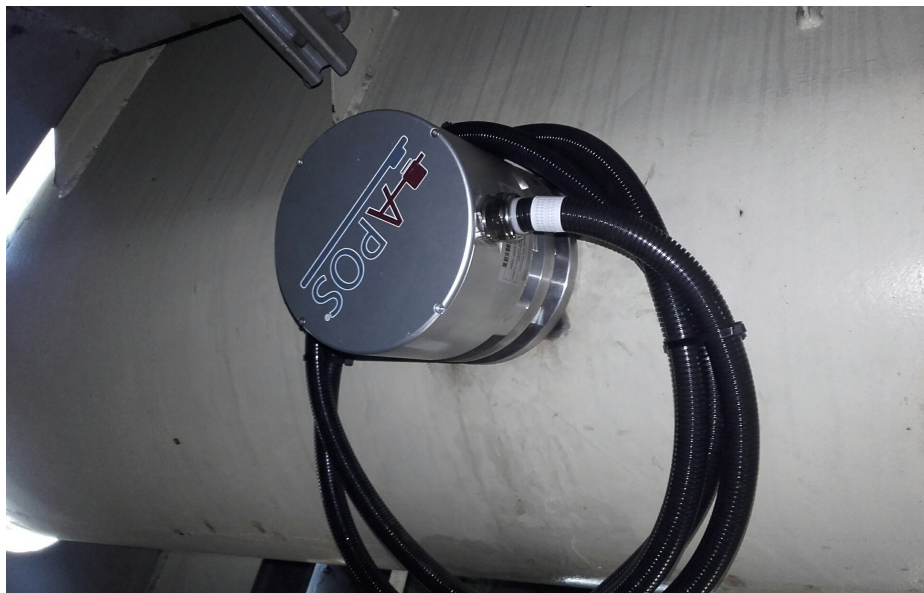
Figure: installation of APOS contact sensor on conveyor screw unloading chip silo in MDF production
