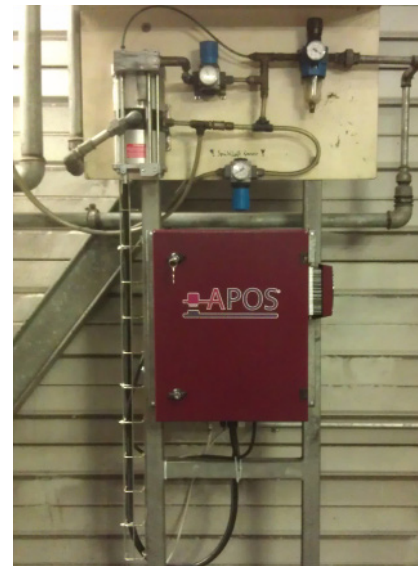
APOS Unit installed in Heiligengrabe
