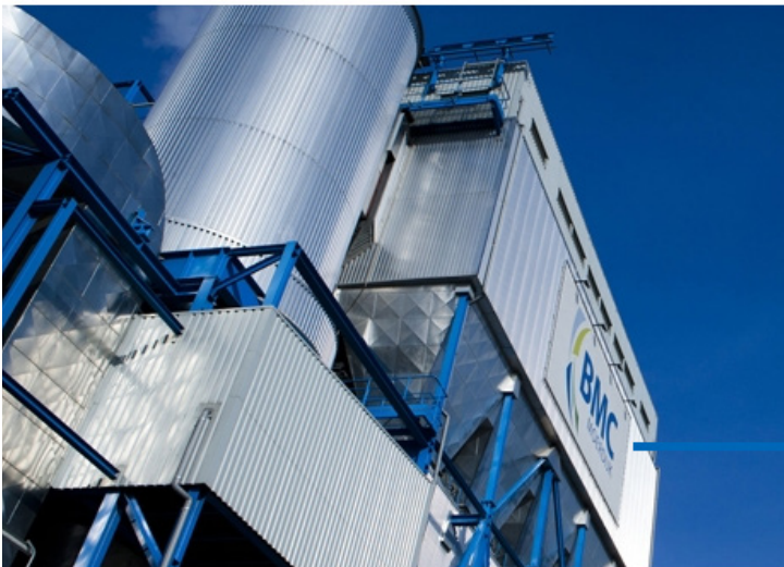
Biomass CHP BMC Moerdijk
