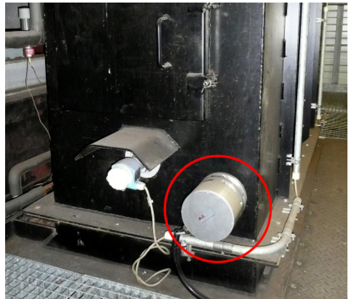
APOS probe installed
