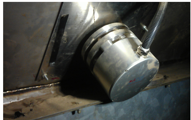
APOS probe installed
