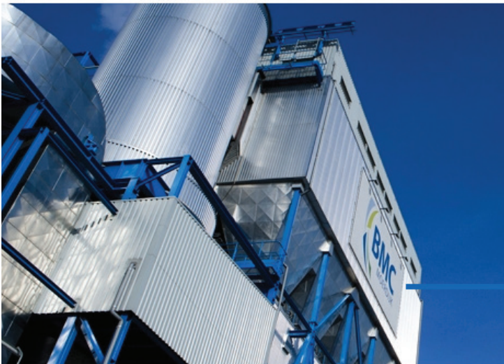
Biomass CHP BMC Moerdijk
